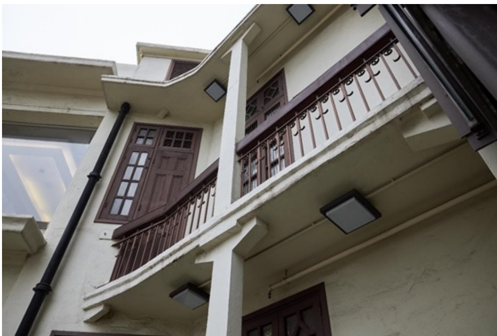
Rear verandah, supported by concrete beams, with the same pattern of railing.
