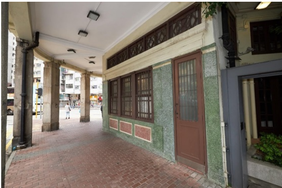
With granite columns supporting on the ground floor, the verandah extends over the public pavements forming arcades.
