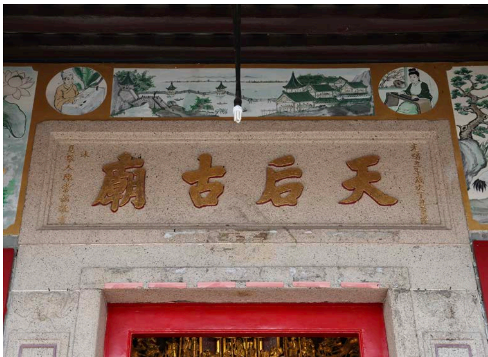
The granite lintel dated 1877 at the main entrance of Tin Hau Temple, Joss House Bay
