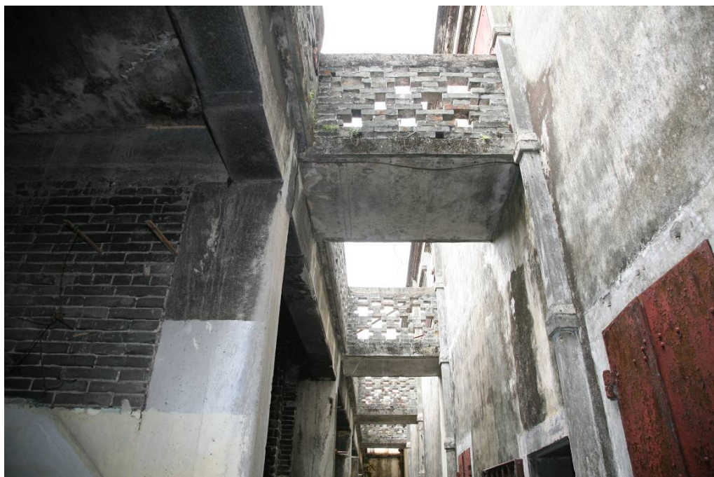
The brick bridges connecting the upper floor of the main building with the roof terraces of the rear outhouses
