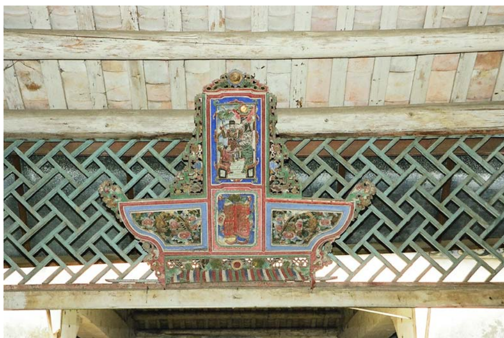
A caimen decorated with carvings of auspicious motifs and Chinese folklore atop the entrance hall
