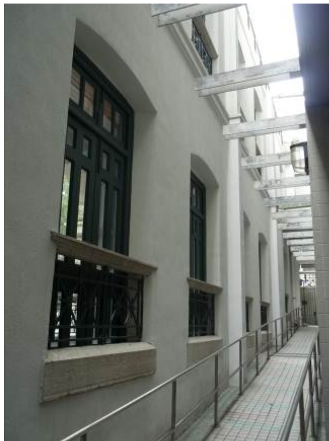
View behind the façade showing the inner skin of the old wall on the left, with the original window openings still intact.
