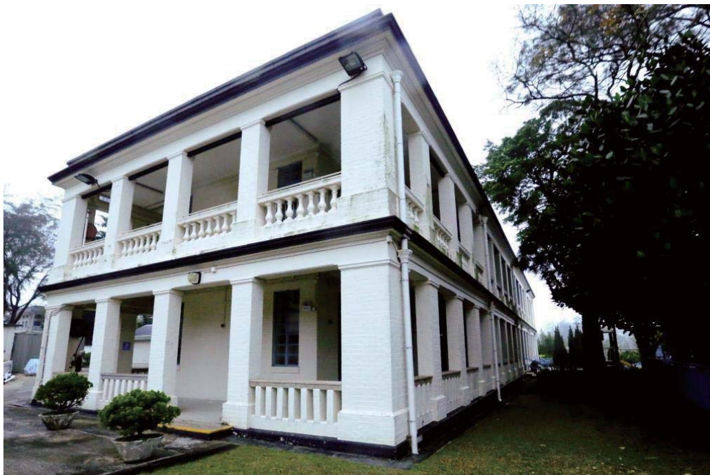
The south facade, of the same design as the east, with urn-shaped classical balustrating on the first floor verandahs.
