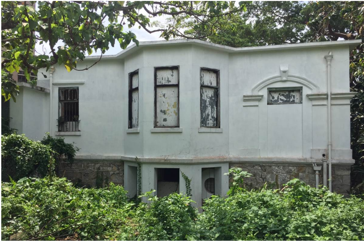
Existing Condition of the Old Dairy Farm Senior Staff Quarters 舊牛奶公司高級職員宿舍的現貌
