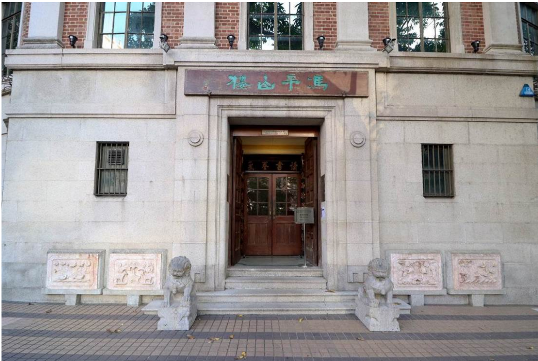
Close view of the front entrance Carved granite doorway is decorated with elegant Classical surround
