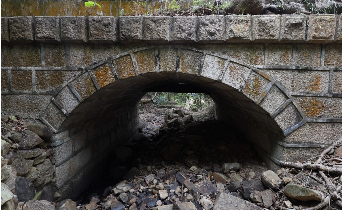
Close view of the Masonry Bridge. The Masonry Bridge is neatly finished with granite copings with chamfered margins and reticulated surfaces.
