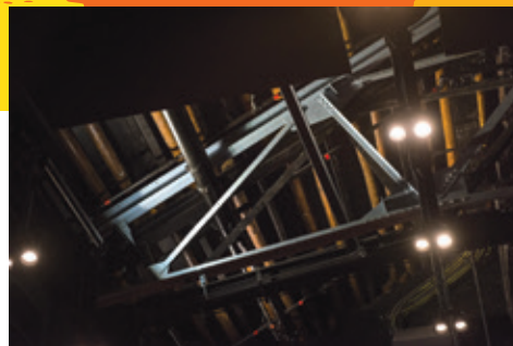
鋼桁架系統和杉木樑條均被保留。 The steel trusses and Chinese fir purlins have been retained.
