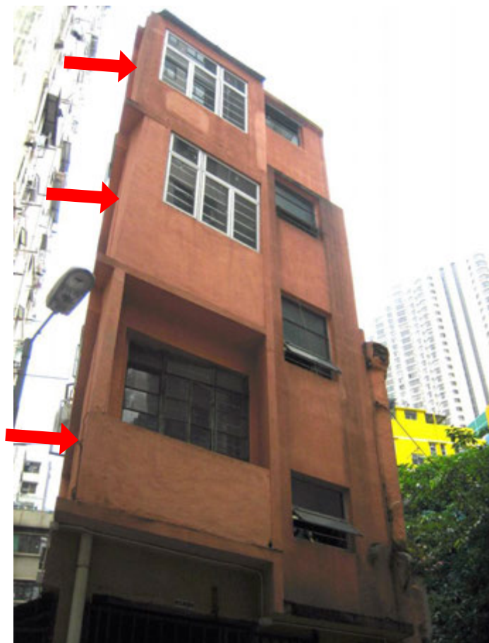
Unauthorized balconies and projecting structures on the first, second and third floor (indicated by red arrows)
