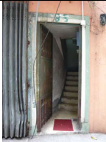
3.2) Main Entrance - Terrazzo 'two-tone' treatment around the frame of the entrance door
