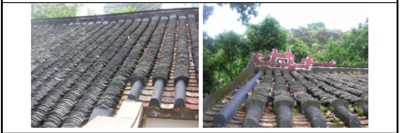
1.6) Chinese style tiled roofs and the geometric motifs at the front and rear ridge-ends at the roof
