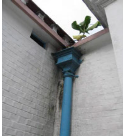
1.10) Cast iron drain pipe and hopper head, located outside the Cell Unit at Rear Wing
