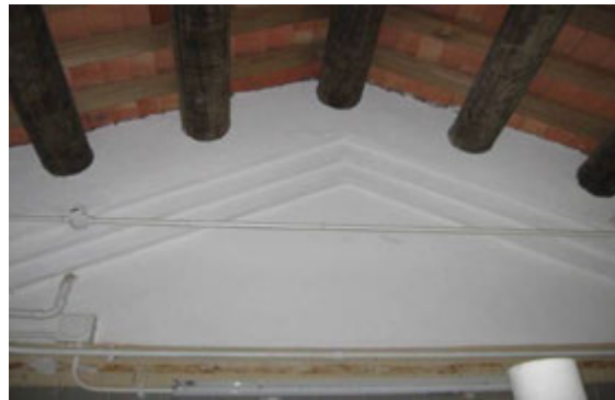
1.8) Plaster mouldings to gable wall of the roof of the North Wing
