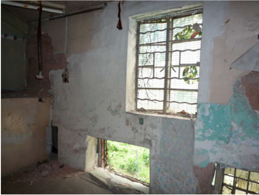
Dilapidated windows on the first floor viewed from the interior
