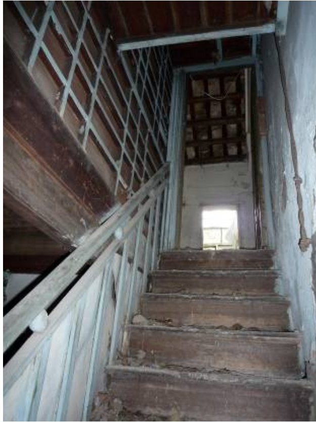
View of the internal timber stair at 31 Hau Wong Temple New Village
