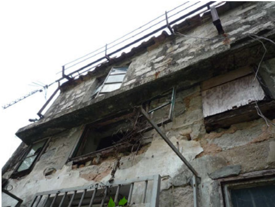
Dilapidated windows on the first floor viewed from the exterior
