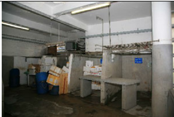
4.6) Open stalls at 1/F with concrete benches and Shanghai plaster dado walls.
