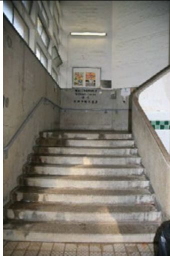
4.4) Staircase, landing and balustrade wall and steel tubular handrail leading from G/F to 1/F
