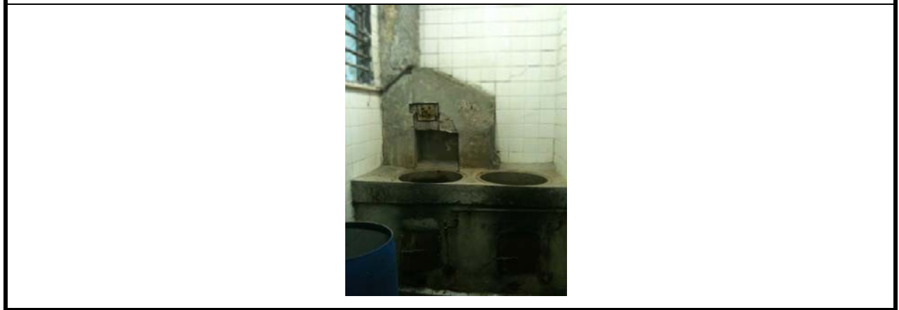
4.2) Stoves and chimney in poultry slaughter room
