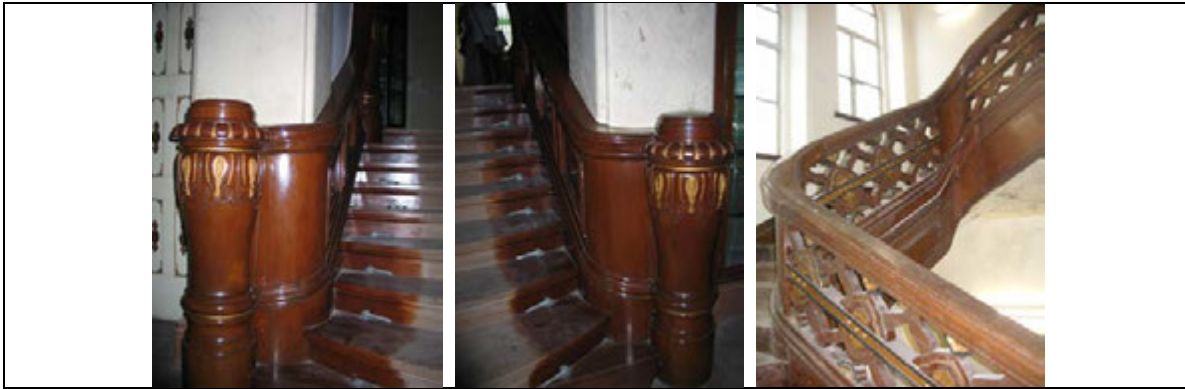
00247 Handrail and guard of the staircase from the ground floor through to the roof floor
