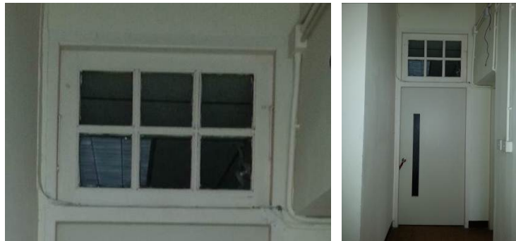
2.2) Timber fanlight and the door frame of the door opening. (The door panel is not original.)
