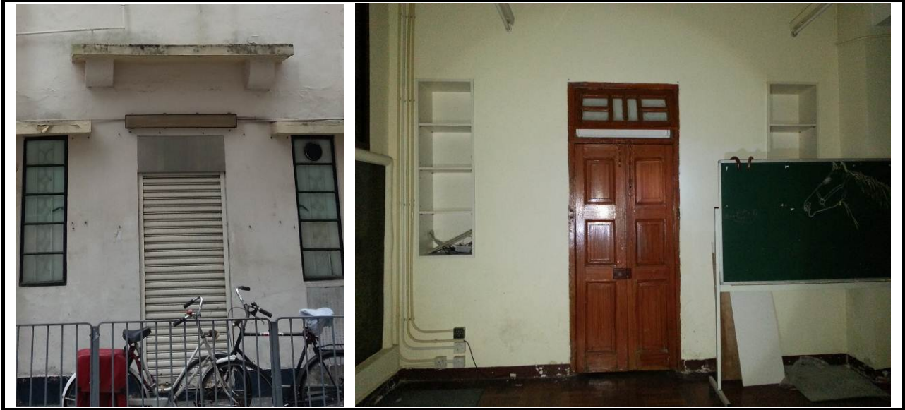
1.3) Timber entrance door and the projected canopy at the main entrance at G/F level. (The metal shutter is not original.)
