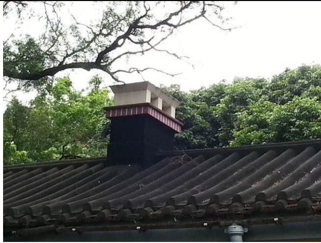
2.7) Chimney stacks with ornamental band painted in red and white brick lines.
