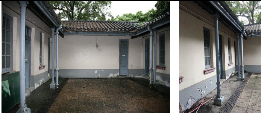
2.8) Open courtyard of the Bungalow including cast iron columns with concrete plinths supporting the roof eaves.
