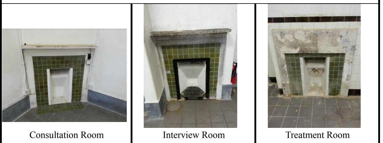
1.12) Fireplaces (3 Nos.) in the Consultation Room, Treatment Room and Interview Room, including tiling, surrounds, grates, hearths and mantel shelf.
