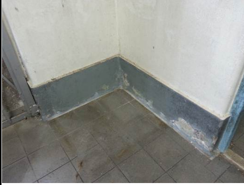
1.16) Original cement skirting.
