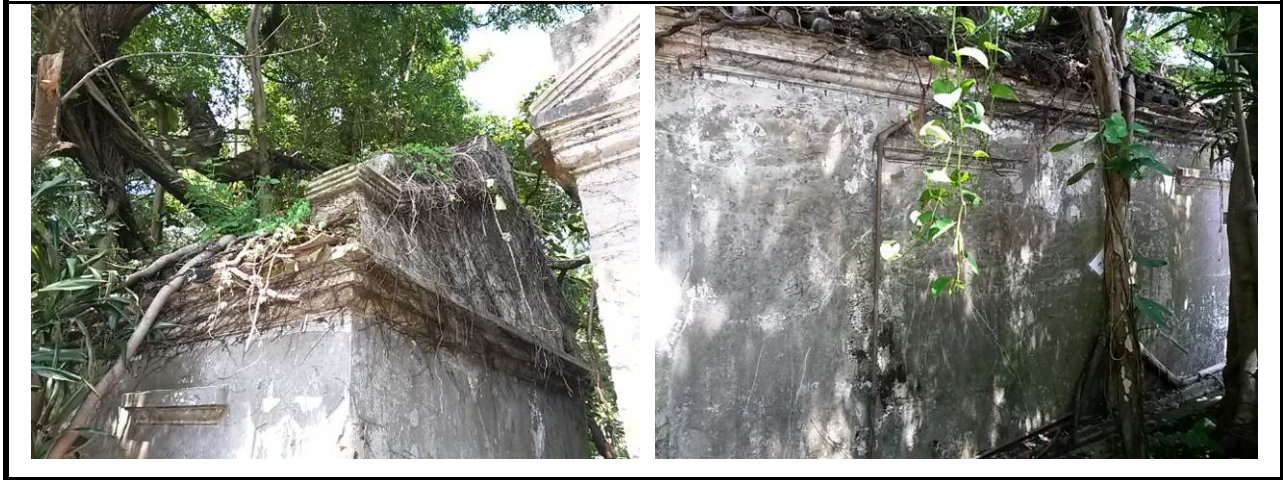
3.3) Moulded copings and horizontal moulded bands to the pitched roof, and the moulded canopies of the blocked door openings at the Servants' Quarters
