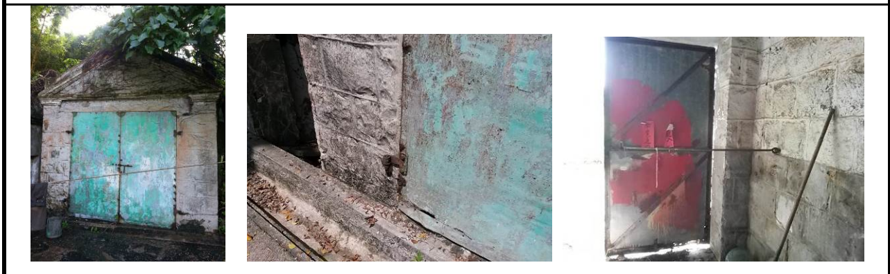
3.5) Door opening at the Garage Block, including the door hinges and the door stay
