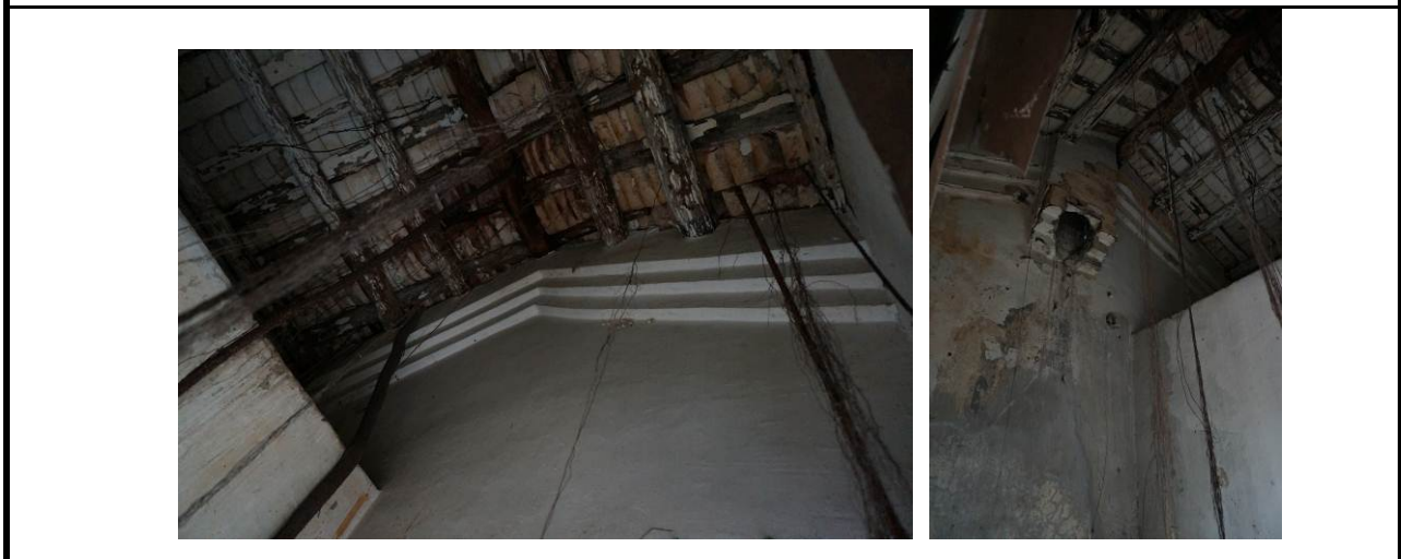
3.4) Corbelled mouldings to the roof and the remains of chimney at the Servants' Quarters
