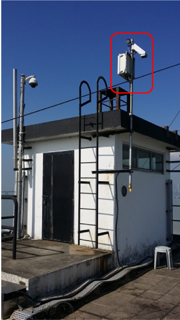
Existing HKO's instrument (lightning sensor) on Roof
