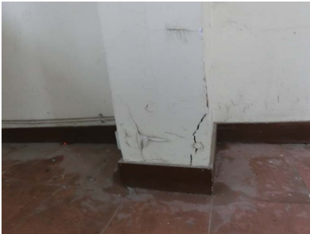
Example of Spalled / Cracked concrete on column in Report Room on G/F
