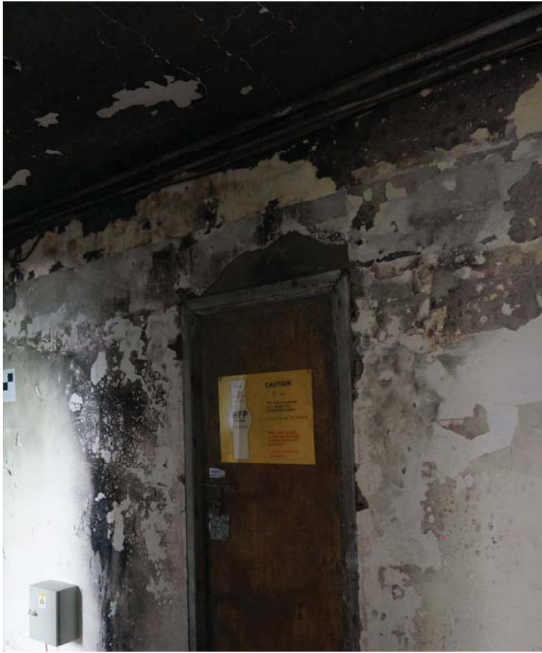
Sign of fire incident in the corridor
