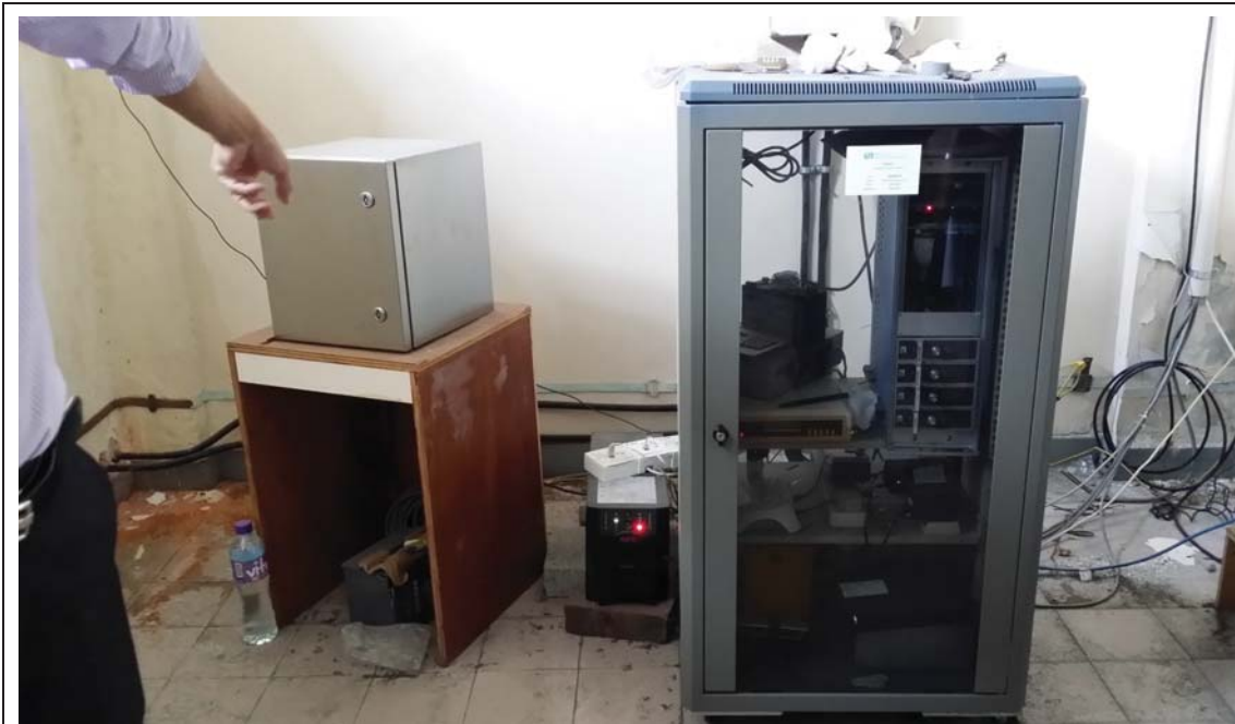
Existing HKO's data acquisition and transmission equipment on 1/F
