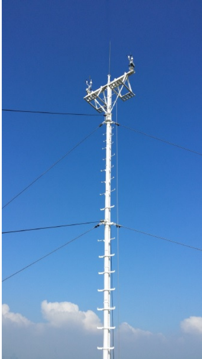
Existing HKO's instruments (anemometers (wind sensors) and its mast) on Roof
