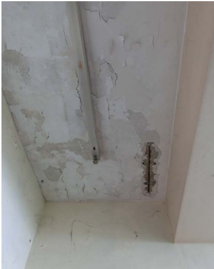
Example of Spalled / Cracked concrete on ceiling in Report Room on G/F
