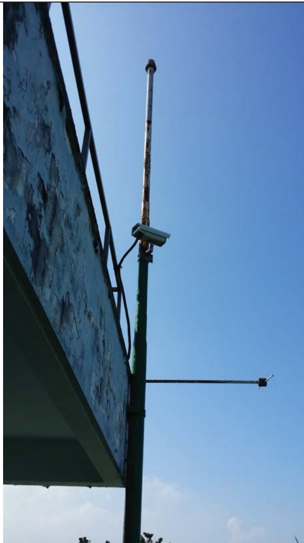
Existing HKO's Equipment (weather camera) on Building Elevation facing North
