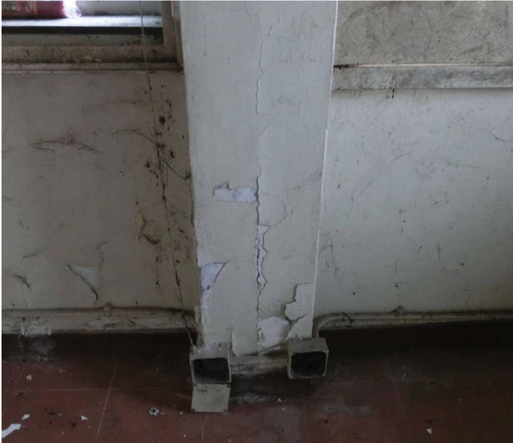
Example of Spalled / Cracked concrete on column in Report Room on G/F
