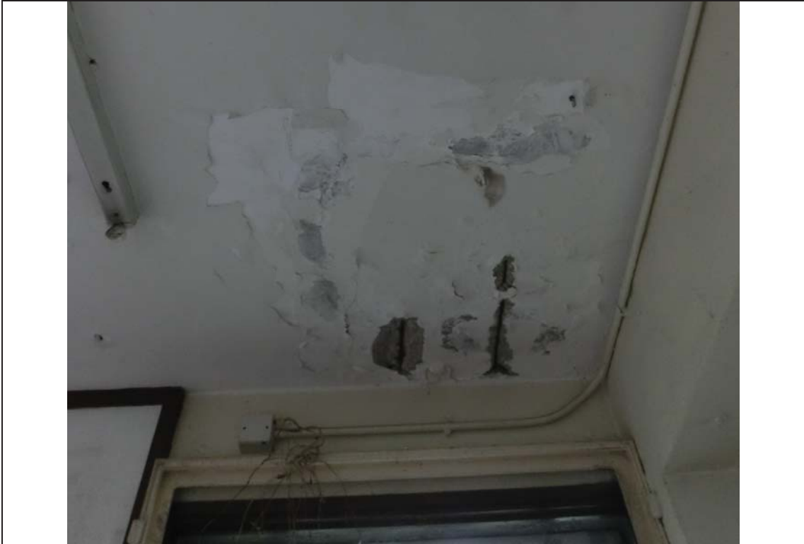
Example of Spalled / Cracked concrete on ceiling in Report Room on G/F
