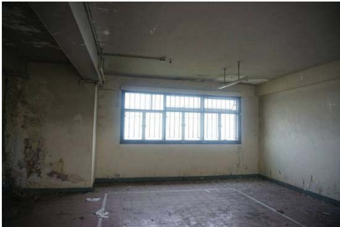
General View of Rest Room / Briefing, Operation Room and Conference Room at 1/F
