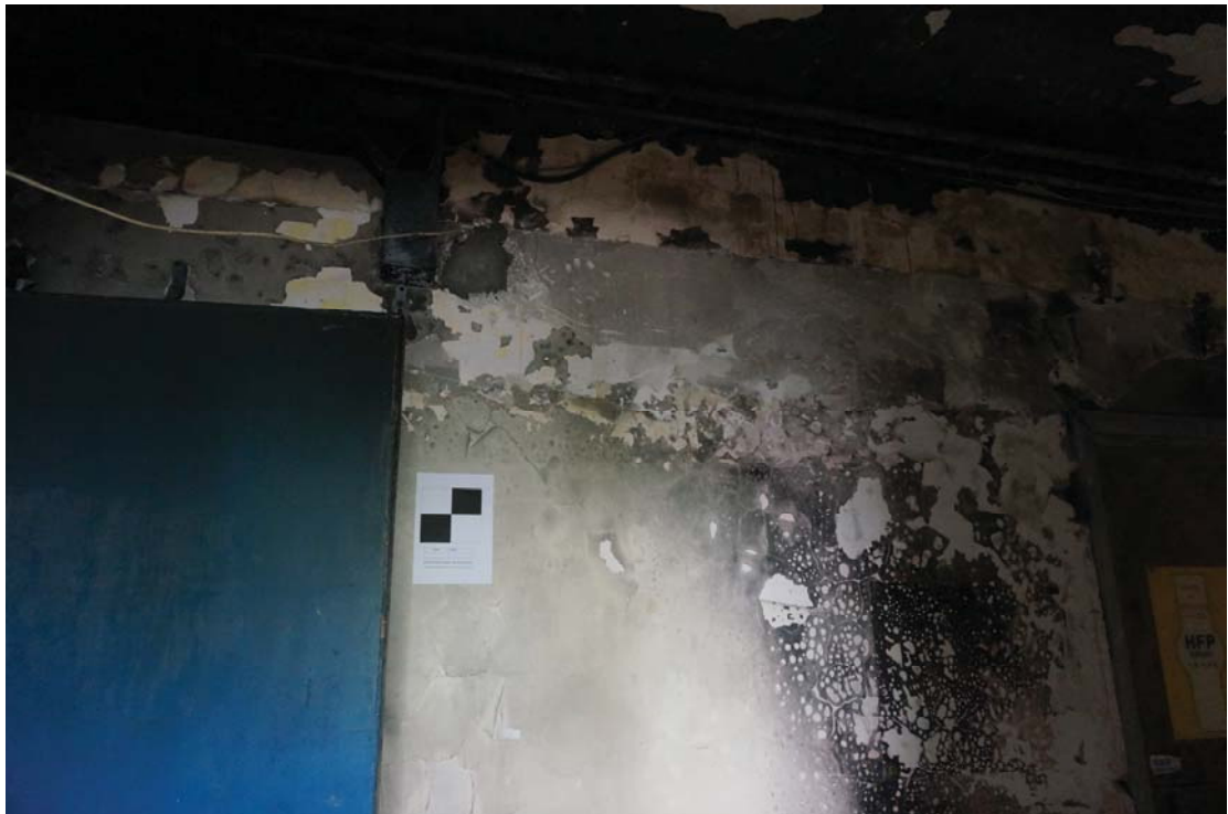
Sign of fire incident in the corridor
