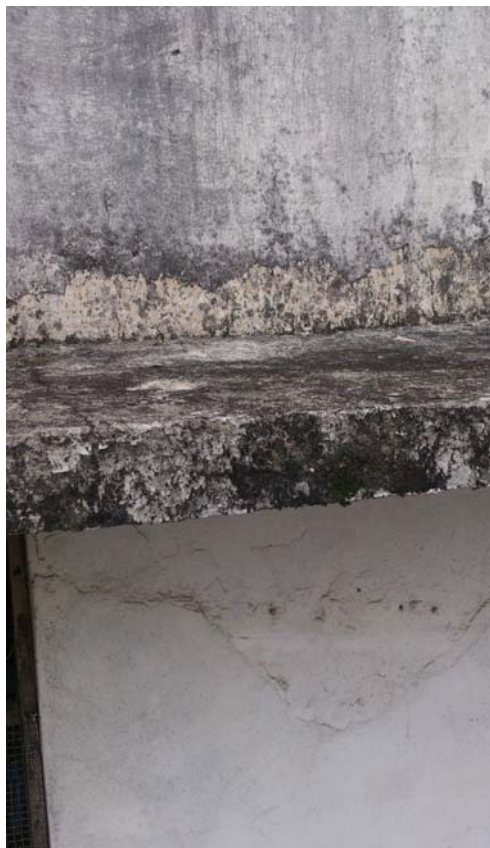
Photo 22 Example of the slight crack on canopy
