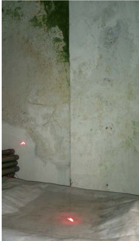
Photo 21 Example of the leakage of roof
