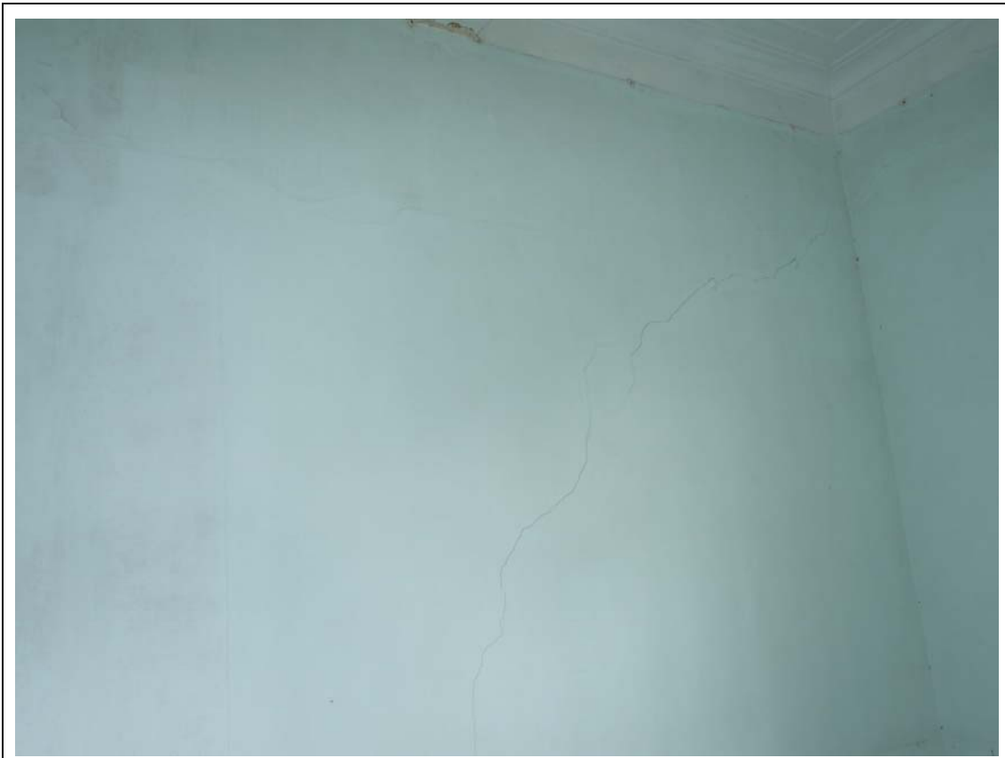
Crack on brick wall at 2/F
