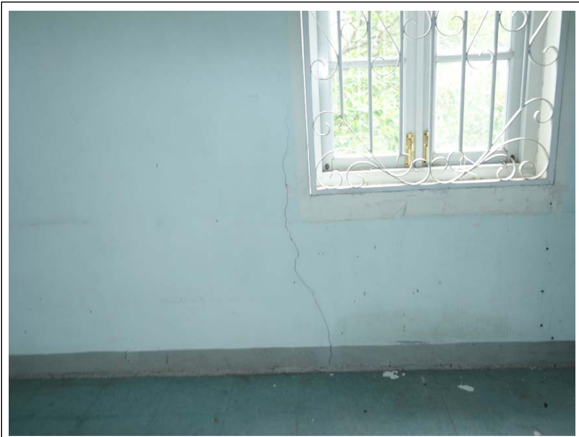
Crack on brick wall at 2/F
