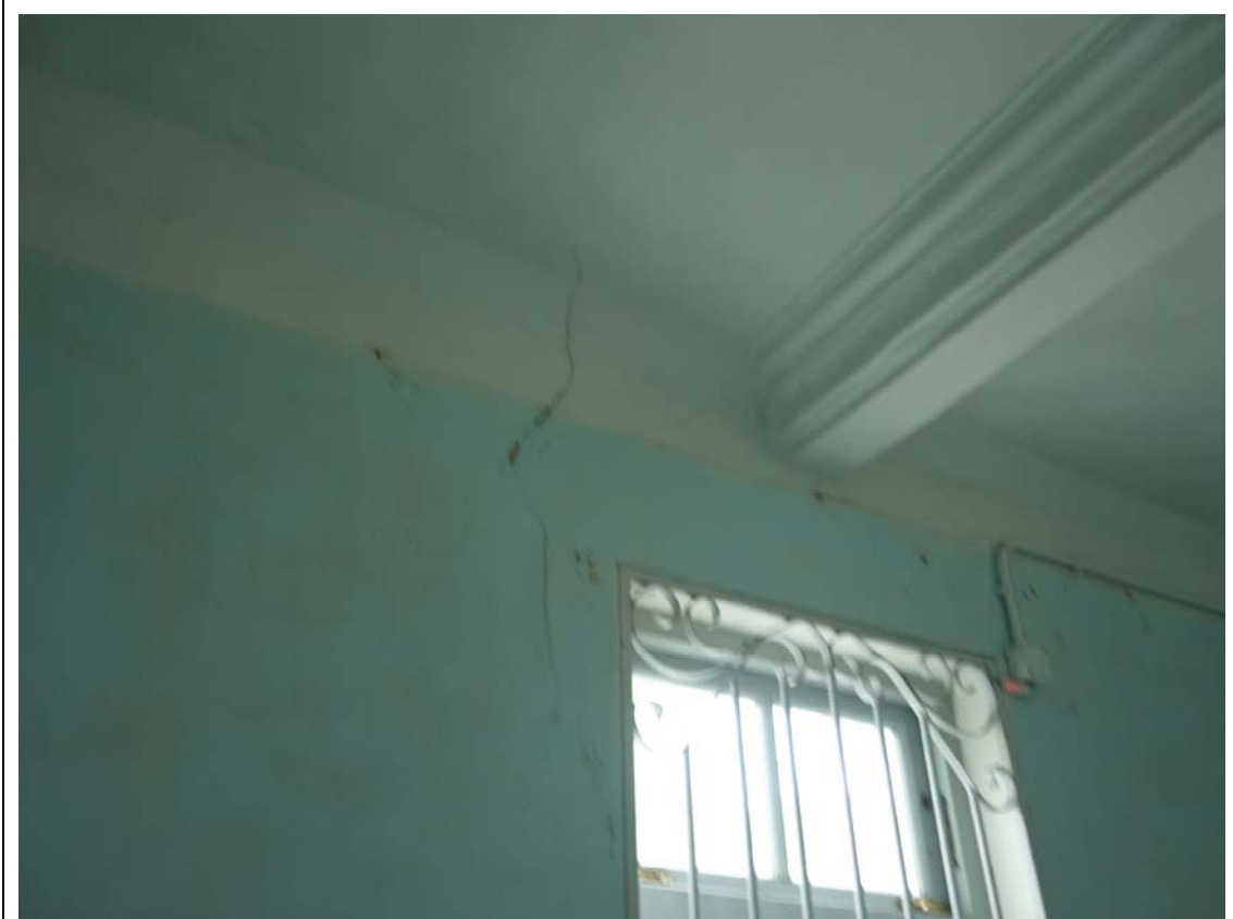
Crack on brick wall at 1/F
