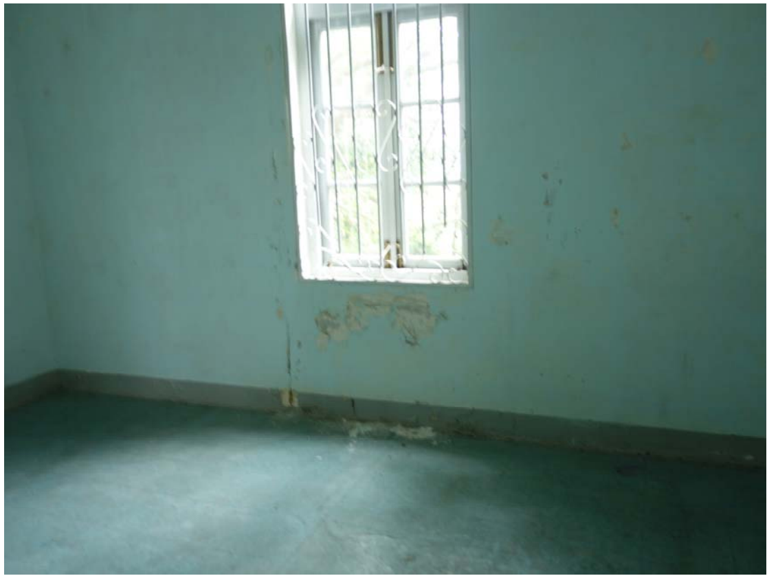
Crack on brick wall at 1/F
