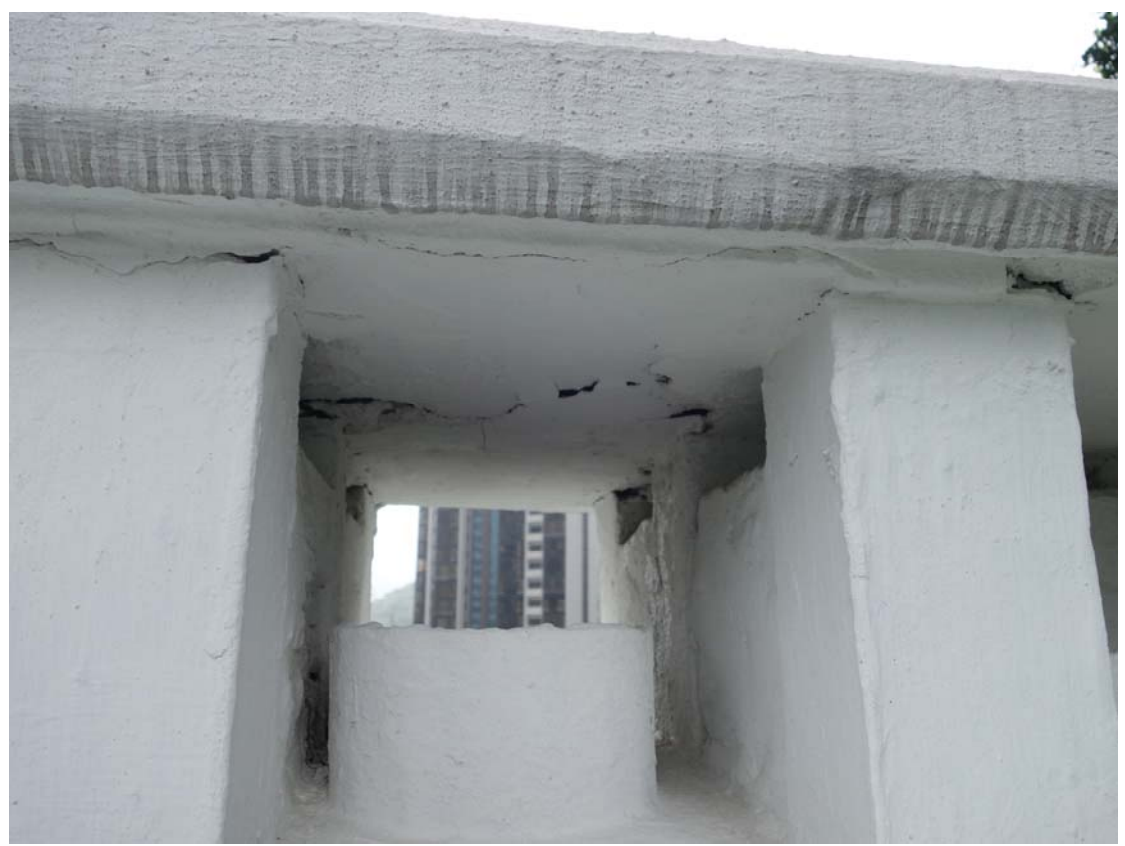
Spalled concrete on the chimney capping
