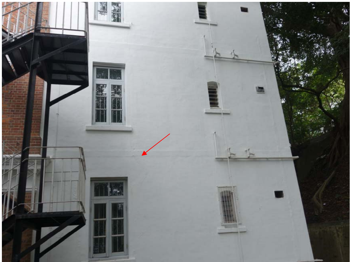
Crack on brick wall from G/F to 2/F
