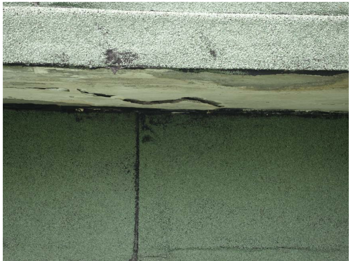
Spalled concrete on the roof eave
