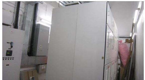
Existing Main Switch Room
