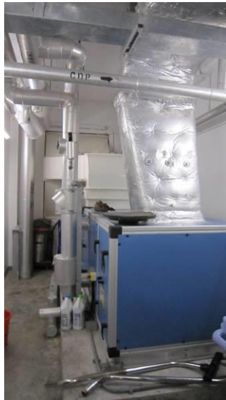
Existing PAU Room
