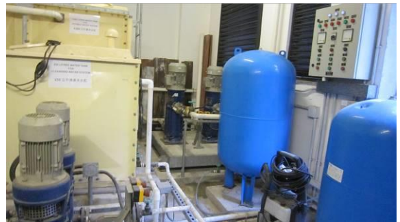
Existing Fresh Water Pump Room
