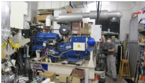
Existing Emergency Generator Room
