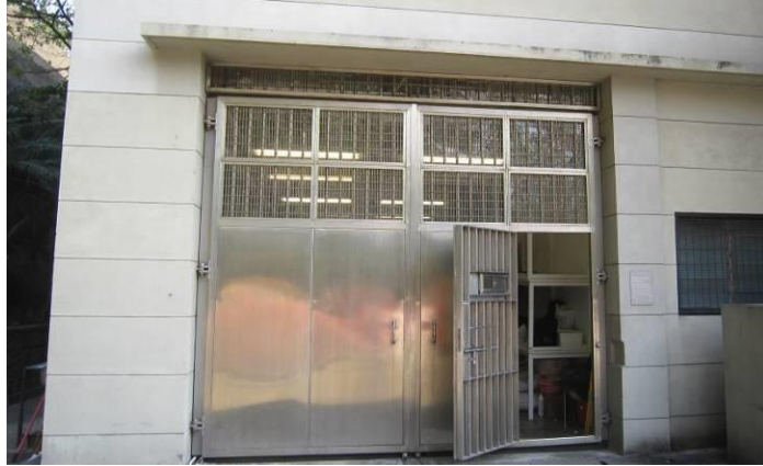
Original wall opening for the old Police Van Garage with old metal gate
