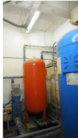
Existing Flushing Water Pump Room
