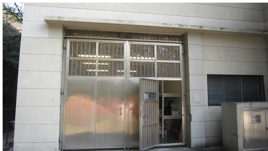
Original wall opening for the old Police Van Garage with old metal gate
