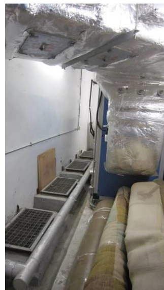
Ducts Room (Grid D-F)
