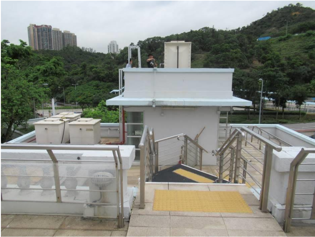
View of Roof & Upper roof (Photo taken at roof of Main Building)
