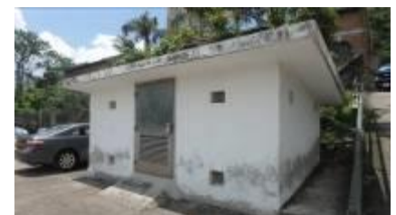
Dangerous Goods Store
