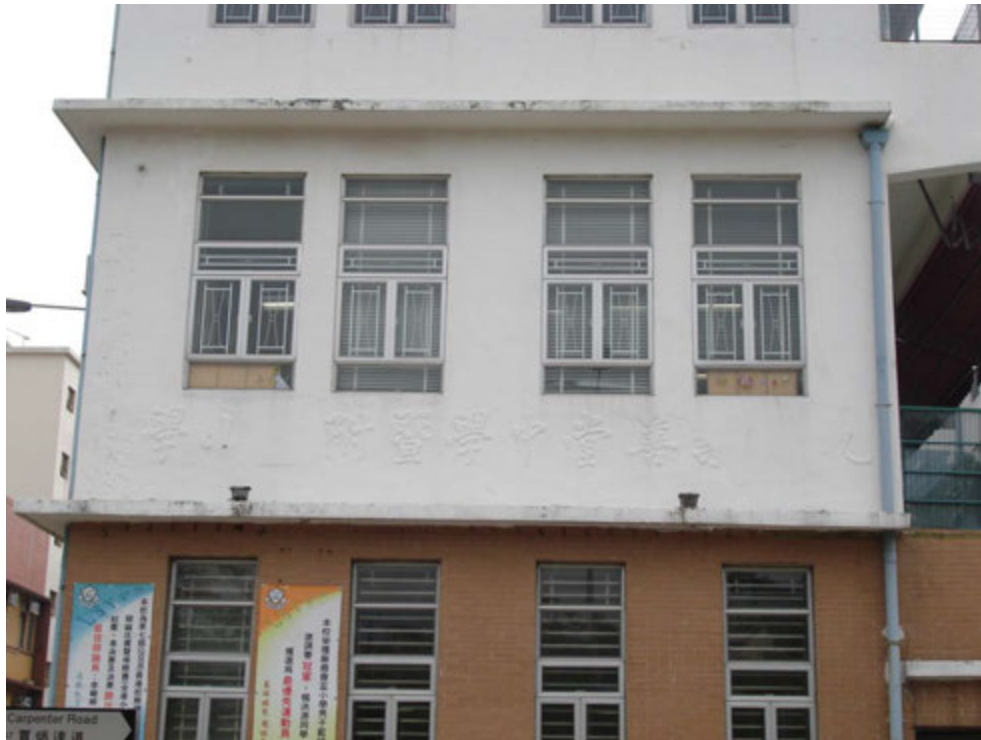
Fig. 221. Inscription of the original school name on the façade facing Carpenter Road.
