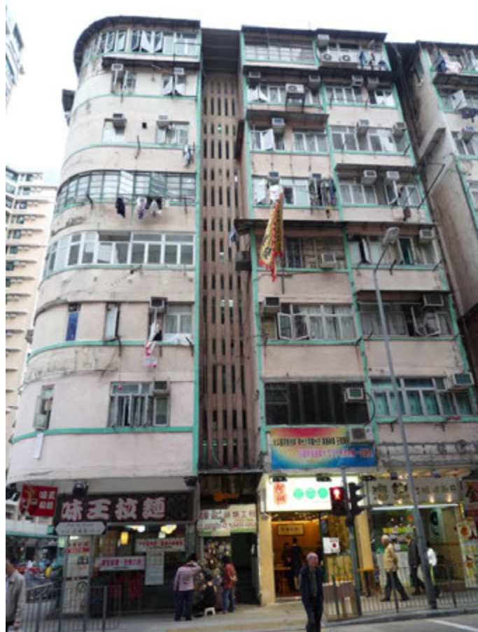
Fig. 296. Staircore with ventilation grilles at the front elevation of Nos. 38-40A Pak Tai Street.
