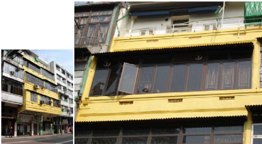
Fig. 251. Mouldings and patterned metal grilles at the parapets of Nos. 18-20 Junction Road.
