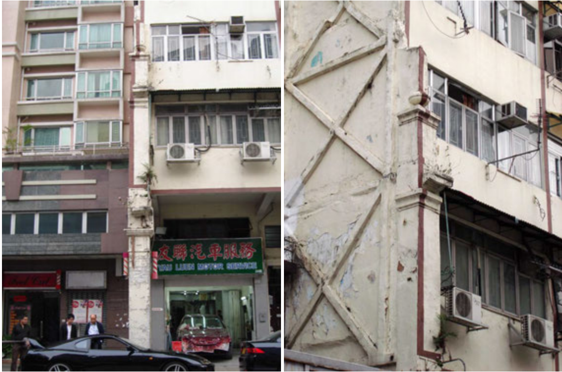
Fig. 294. The remains of the column of a tenement house at No. 20 Pau Chung Street.
