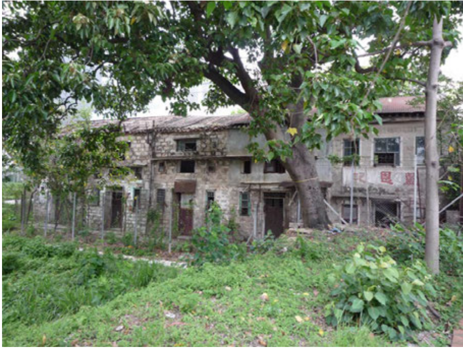
Fig. 243. Front view of the Stone Houses at No. 31-35 Hau Wong Temple New Village
