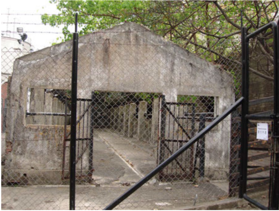
Fig. 65. Ruinous structures found at the rear of the site nowadays.
