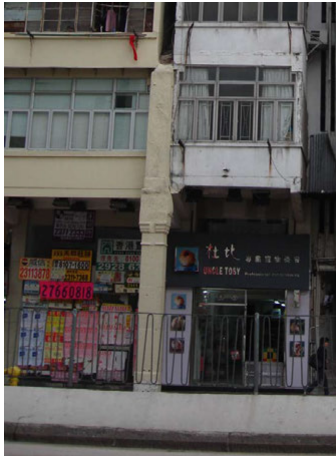
Fig. 295. The remains of the column of a tenement house at No. 324 Ma Tau Wai Road.
