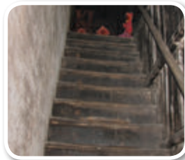
破損的梯級暨板與級面。 Worn-off risers and treads.
