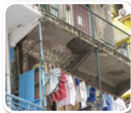
露台破損的混凝土。 Defective concrete at balconies.
