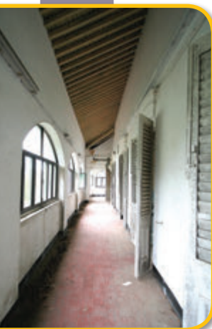
長廊是舊大澳警署的設計風格。 The verandah is a notable architectural feature of Old Tai O Police Station.
