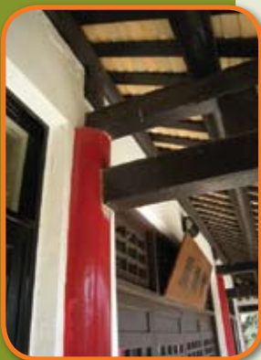
道風山基督教叢林「會議廳」結構 Structures of Conference Hall, Tao Fong Shan Christian Centre
