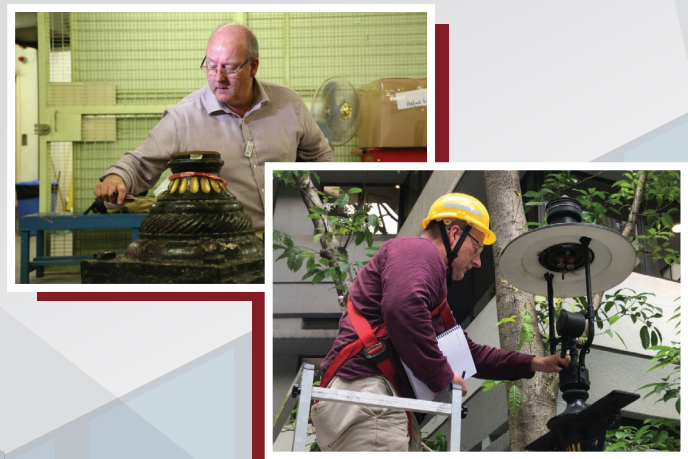
煤氣路燈英國原供應商的專家Mark Jones來港，詳細檢查損毀的煤氣路燈。 Mr Mark Jones, an expert from the original gas lamp supplier in the United Kingdom, came to Hong Kong to conduct a detailed inspection of the damaged gas lamps.
