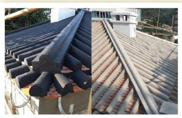
主樓屋頂曾被改動，由原本的斜屋頂改為平頂，修復工程會盡力把它還原。 The original pitched roof of the Main Building was changed to flat roof in the past, and the rehabilitation works will strive to restore it.
