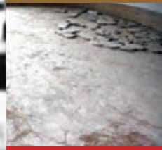
修復前 Before restoration
