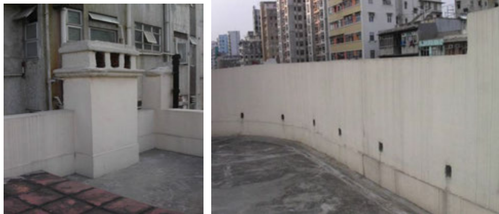
1.11) The brick chimney flue, water tank and parapet completed with drainage outlets
