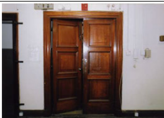
6.9) Original wooden panelled doors and frames to Police Duty Room, Lavatory and Reception Room, etc
